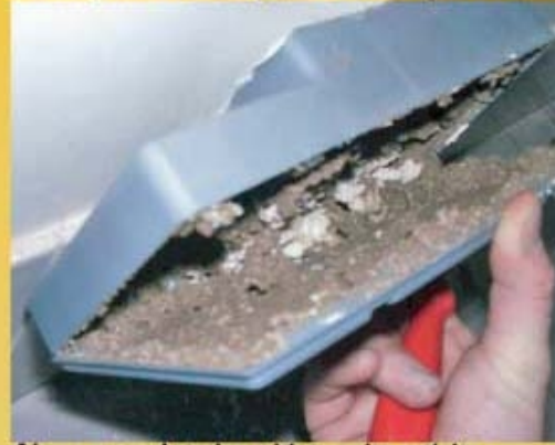
Above ground station with termite activity.
